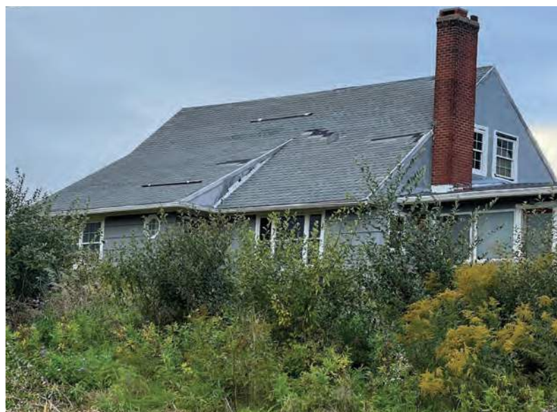
Above: 5 Mountain Edge in Boston Corners is an example of a tax-paid unoccupied home with a beautiful view falling into disrepair. Below, top to bottom: Now being demolished: 145 Farnum Road in Lakeville was purchased in 1964 for $7,000 and after foreclosure eventually sold for $227,000 in January 2026. 86 Upper Main in Sharon, CT will be renovated by new owners. Photos by Christine Bates.
