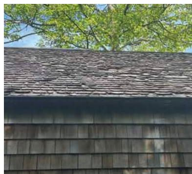
AI analyzed this photo of a cedar roof and concluded “Based on the visual evidence, this cedar shake roof is in poor, failing condition and is at or very near the end of its functional lifespan.”
